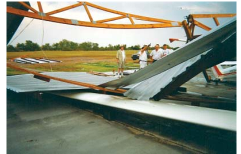
Soaring Club of Houston’s Grob 103 getting a falling girder through a wing was a job for Fred Jiran
